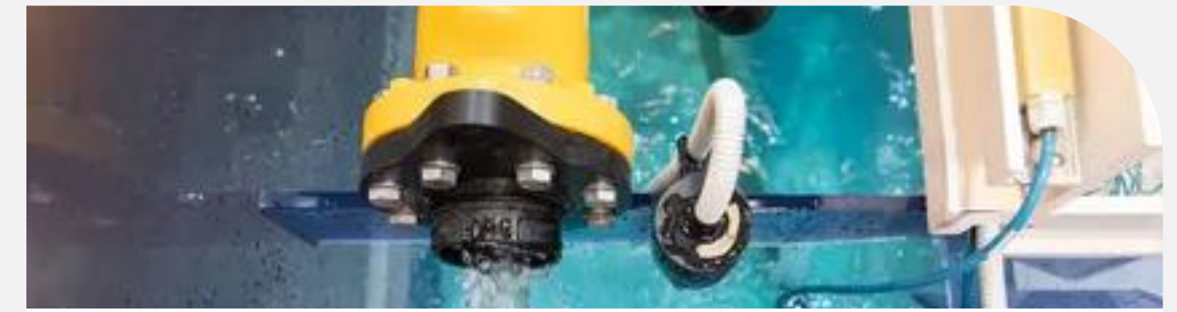
Management of water & sewage plants
